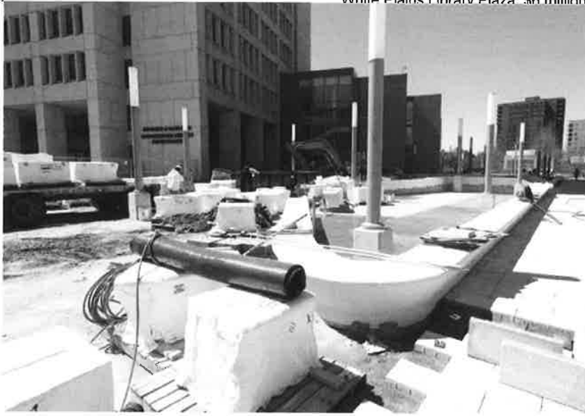
"Seat walls" are pictured as work continues on a multi-million dollar renovation of the White Plains Library Plaza, April 24, 2019. (Photo: Mark Vergari/The Journal News)
